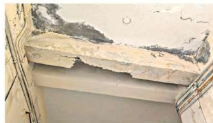
A portion of the roof plaster that collapsed at the Mahatma Gandhi Memorial Hospital in Warangal on Tuesday.
